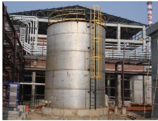
SS TANK FABRICATED AT MEGHMANI
